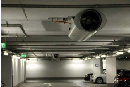
Underground car park with NOVENCO's jet fans AUO 380
